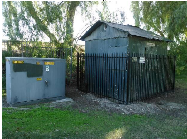
Photo 12 View of the pad mounted transformer on the east portion of the site.
