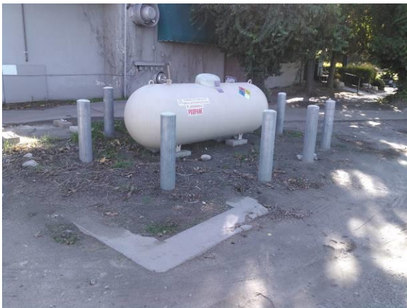
Photo 9 View of the propane AST.
