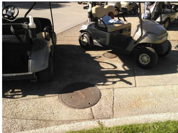
Photo 10 View of the southern septic tank and leach field looking west.
