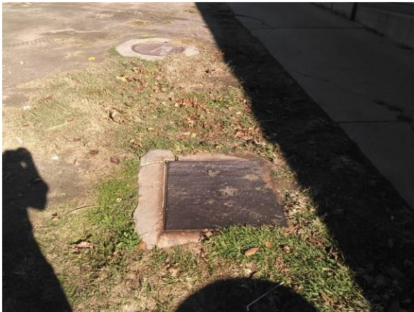
Photo 7 View of the grease trap west of the club house.
